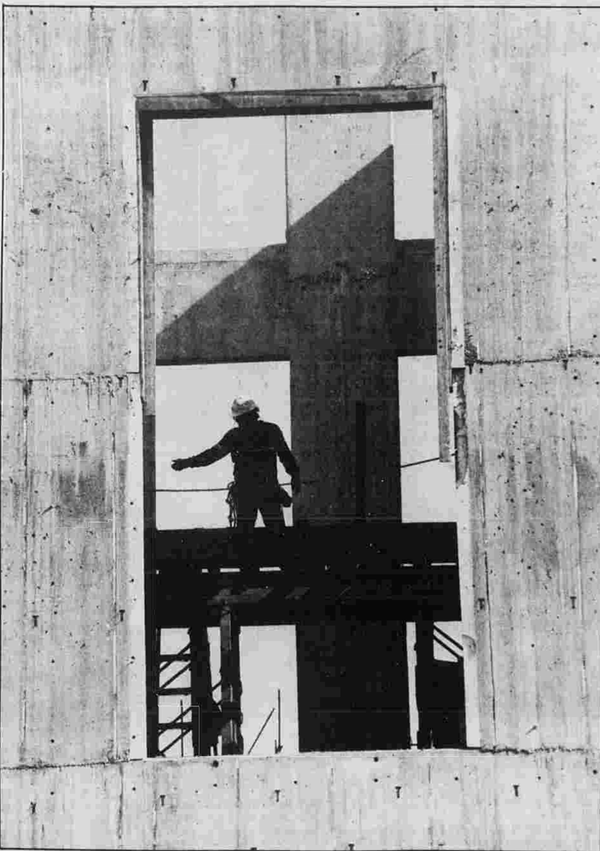
FRAMED — Frank Wadsworth of Caco Concrete Forming Co. puts up girders Tuesday for worker safety in an elevator shaft in what will become a parking garage for Manchester Memorial Hospital.
